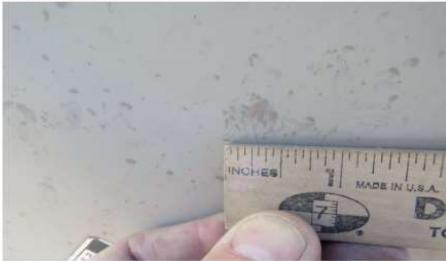
Photograph 26: The northeast, HVAC unit has splash-marks.
