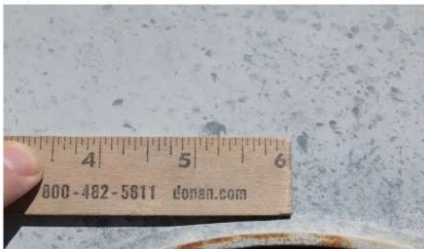
Photograph 6: The electric panel on the south-side of the building has splash marks.
