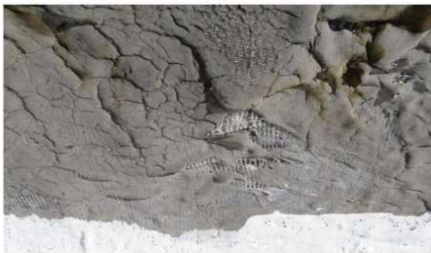
Photograph 30: The vertical sides of the south parapet-wall transition is covered this mastic and have irregular-shaped blemishes with non-fractured fiberglass mat.
