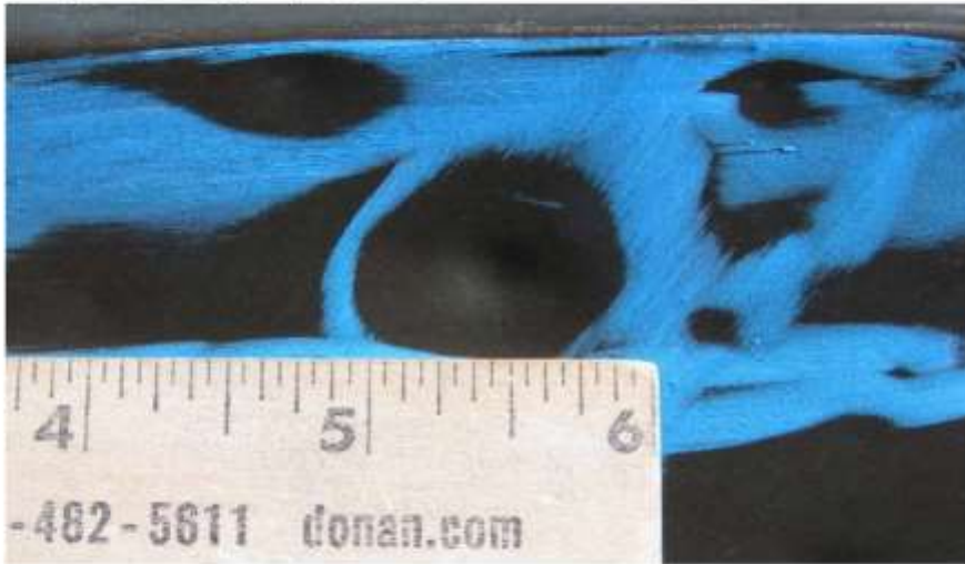
Photograph 12: Close-up of the copper, top-cap flashing that is dented.
