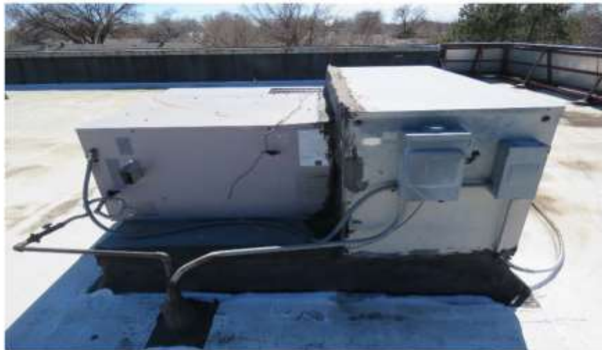
Photograph 23: The southwest, HVAC unit is a 1996 Carrier unit.
