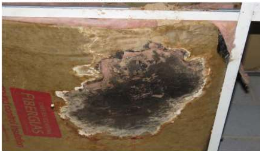
Photograph 46: The batt-insulation above the drop-ceiling is stained black.
