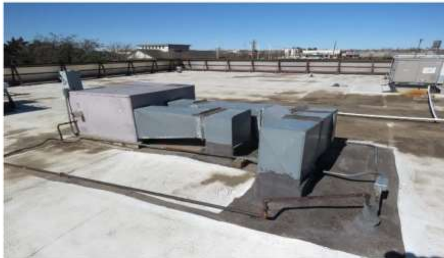
Photograph 21: The middle HVAC unit is a 1997 Carrier unit.
