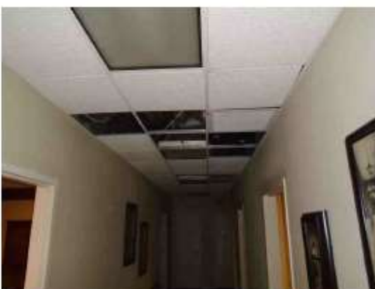
HALLWAY CEILING DAMAGE
