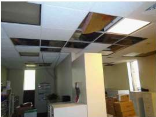
STORAGE/FILE ROOM CEILING DAMAGE
