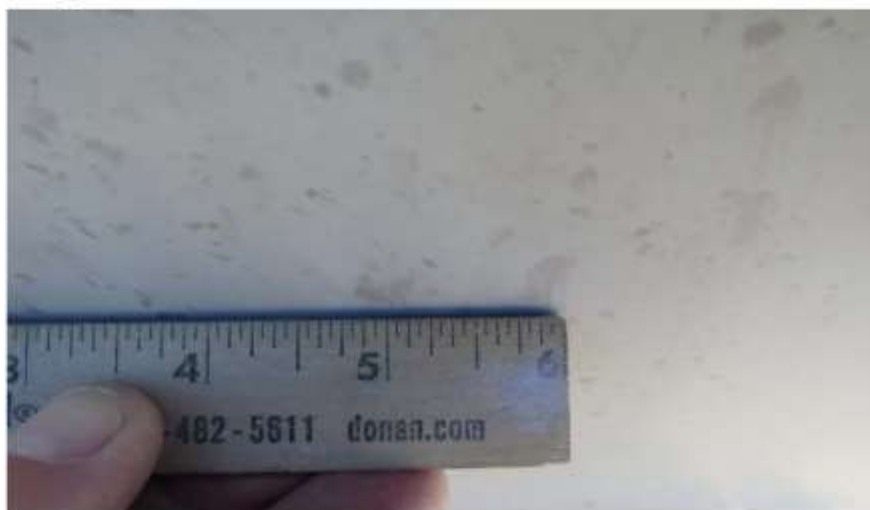
Photograph 22: The middle HVAC unit has splash-marks.
