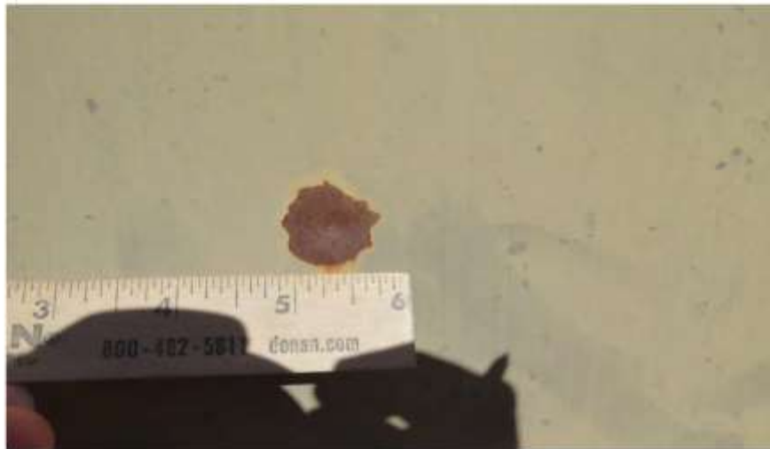
Photograph 7: The south, metal door is rusted at dents.
