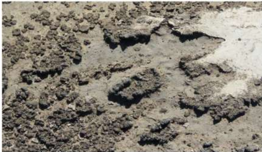
Photograph 43: Remaining mastic and granules in the dark-stained areas of the roof.
