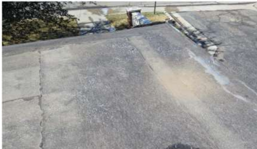
Photograph 37: The non-painted, modified bitumen membrane is missing granules and mastic.
