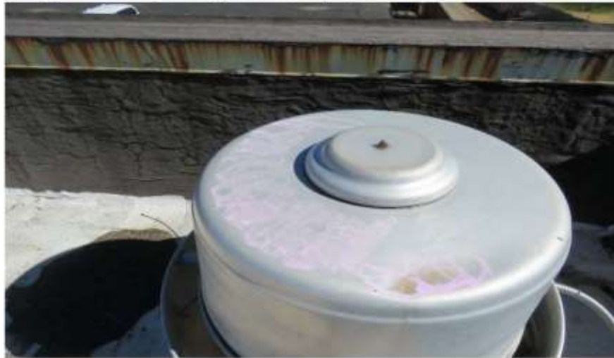
Photograph 16: The top of the powered blower is dented.
