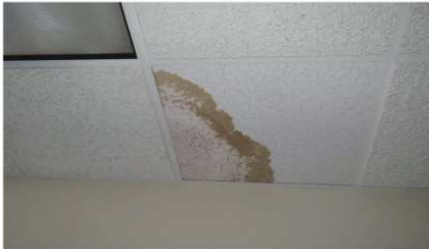
Photograph 45: Alternate example of the ceiling tiles throughout the building have multiple-rings of staining with varying shades to the stains.
