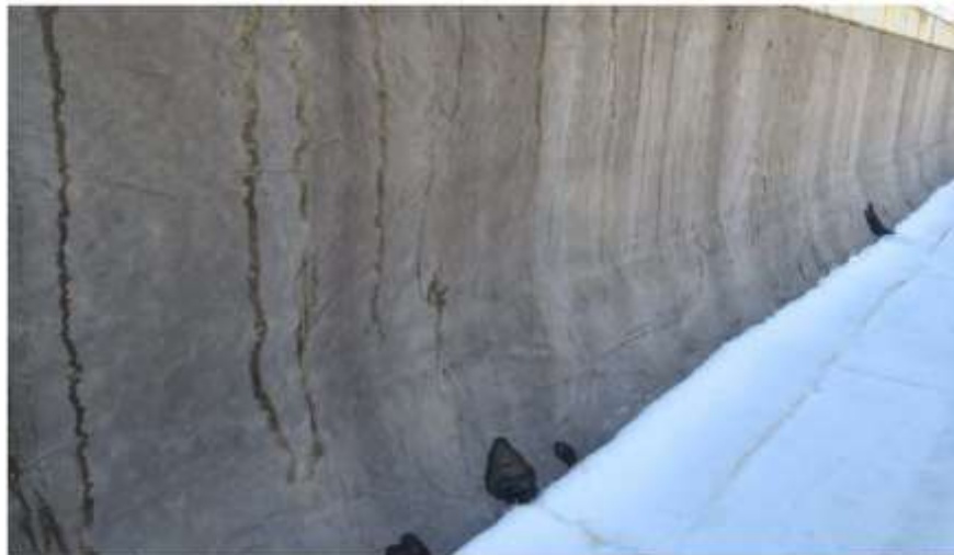
Photograph 29: The vertical sides of the south parapet-wall transition is covered this mastic.
