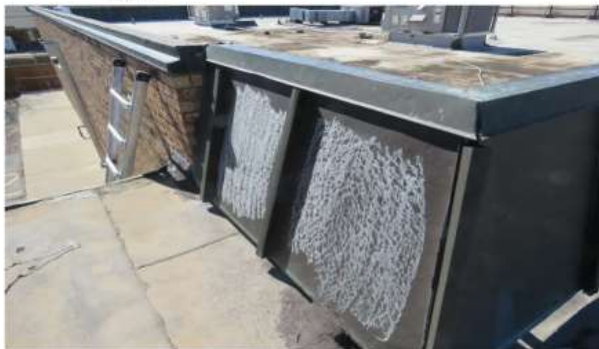
Photograph 14: Copper covered faux parapet walls are dented.
