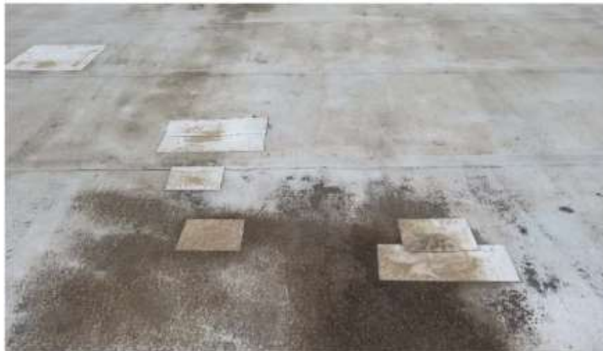
Photograph 41: The roof has previous repairs.
