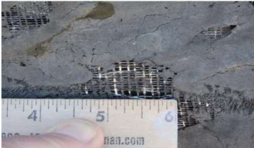
Photograph 28: The tops of the parapet-walls have blemishes with missing mastic no fractures of the mat.
