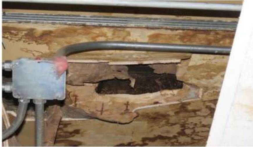
Photograph 47: The reinforced, concrete roof decking is exposed and missing above the interior, drop-ceiling
