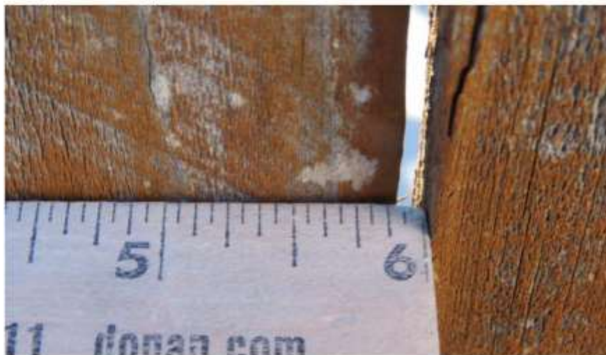
Photograph 10: The south-facing wooden fence has clean marks.
