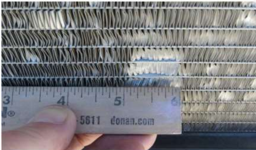
Photograph 20: Close-up of the dented cooling fins on the HVAC units.
