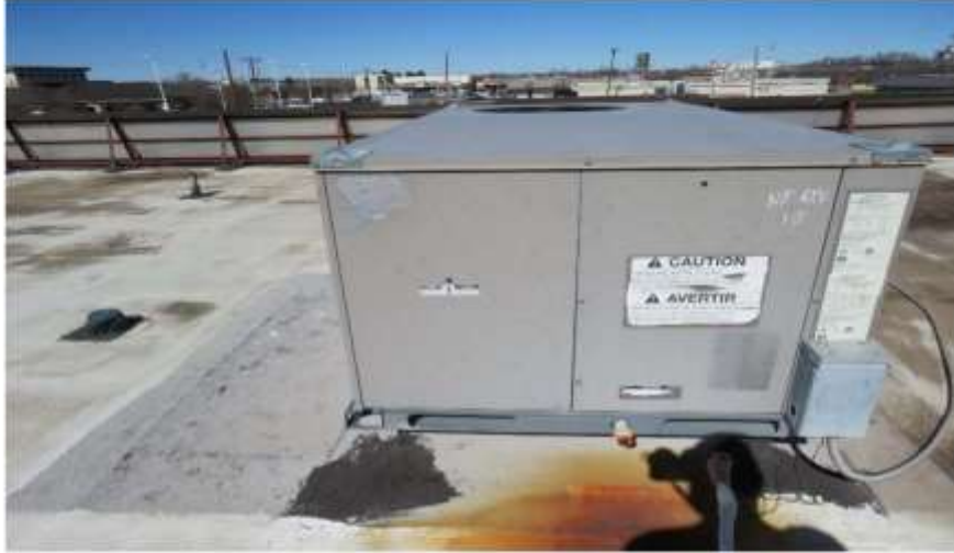
Photograph 25: The northeast, HVAC unit is a 2010 York unit.
