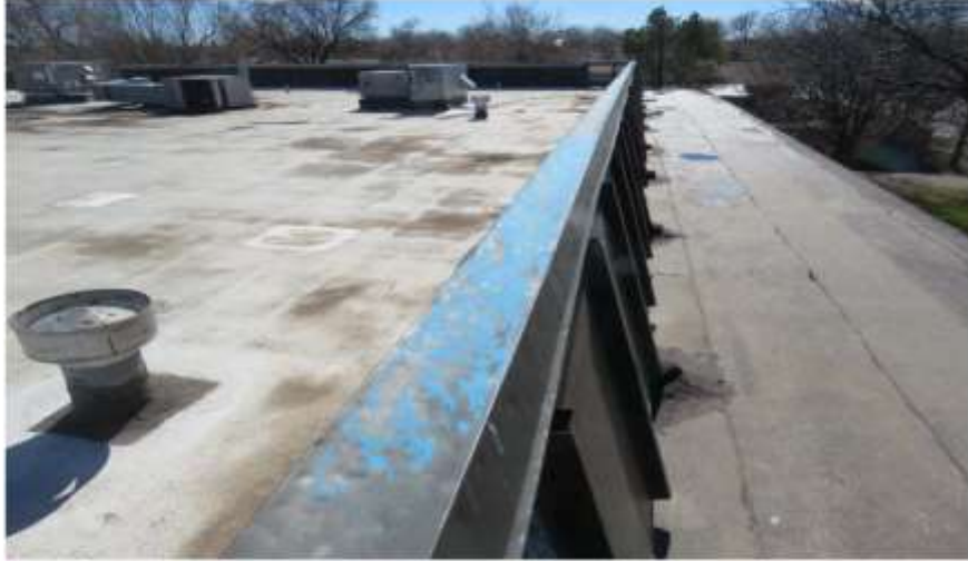
Photograph 11: The copper, top-cap flashing is dented.
