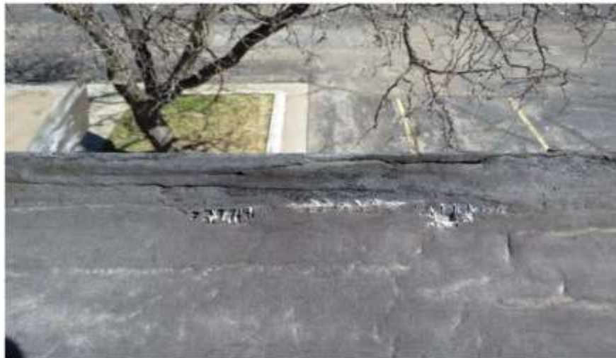
Photograph 31: The top of the east, parapet wall has linear blemishes with missing mastic and fractured fiberglass mat.
