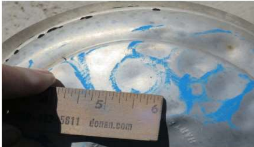
Photograph 18: The tops of the metal flues are dented.
