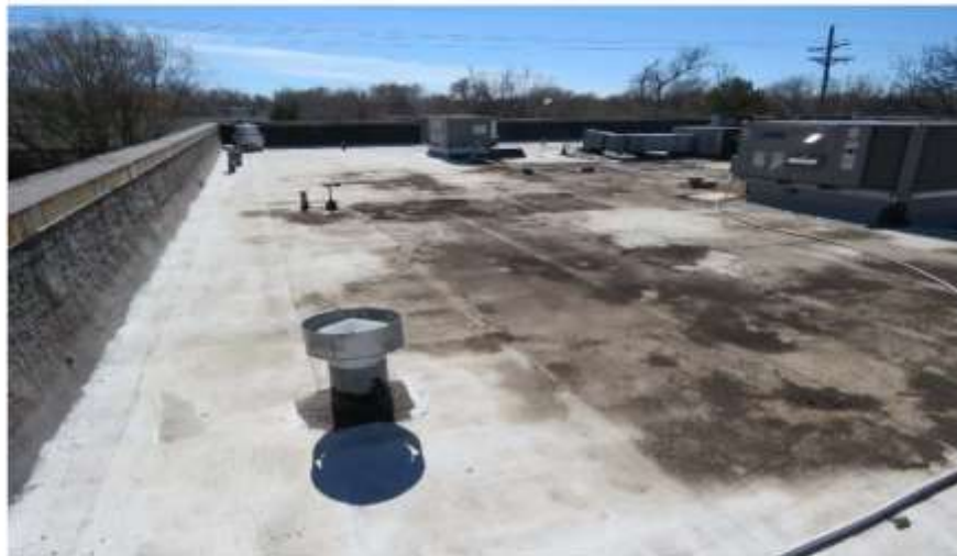
Photograph 39: The paint-covered, modified bitumen membrane has large patches of dark stains with dirt middle of the roof.
