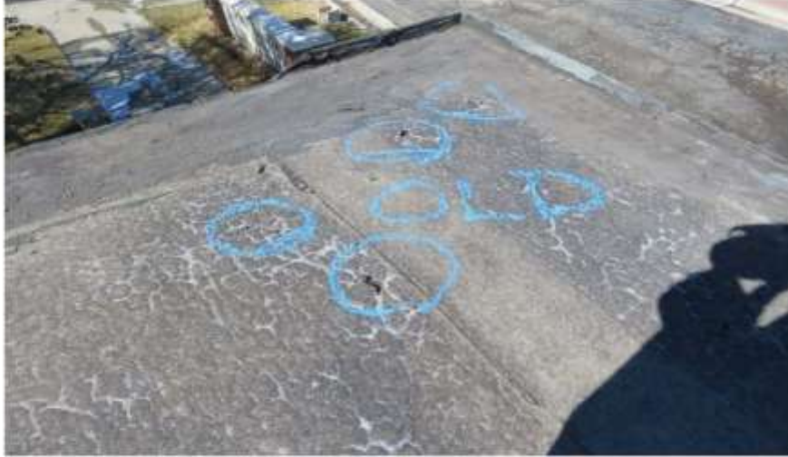
Photograph 35: The non-painted modified bitumen membrane has irregular-shaped blemishes with missing felt paper.
