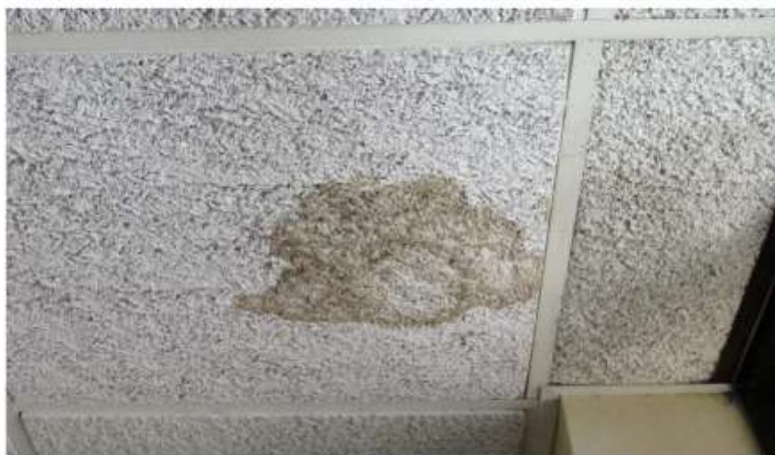
Photograph 44: The ceiling tiles throughout the building have multiple-rings of staining with varying shades to the stains.
