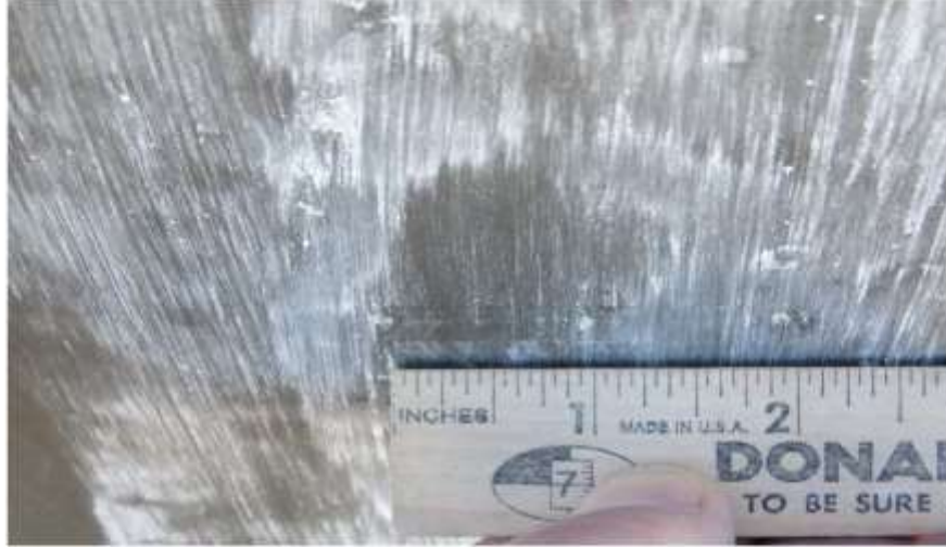
Photograph 15: Close-up of the copper covered, faux parapet walls that are dented.
