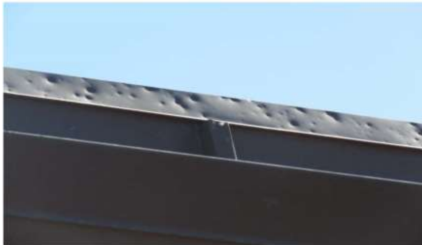
Photograph 9: The copper fascia around the building is dented.
