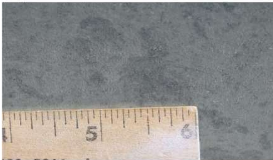
Photograph 24: The southwest, HVAC unit has splash-marks.
