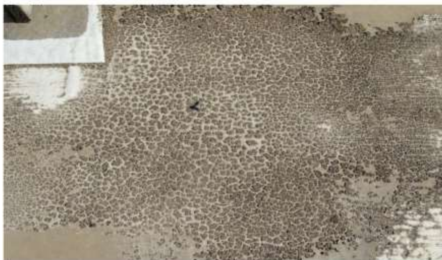
Photograph 42: The paint-covered, modified bitumen membrane at patches of dark stains is delaminating and the mastic is missing.
