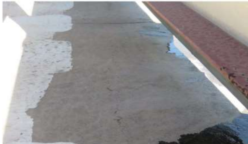
Photograph 33: The modified bitumen roof outside of the copper-paneled, faux parapet walls is not painted.
