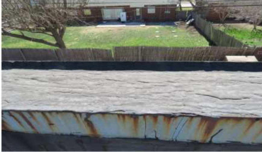
Photograph 27: The tops of the south parapet-walls is covered with a metal top-cap flashing and mastic.
