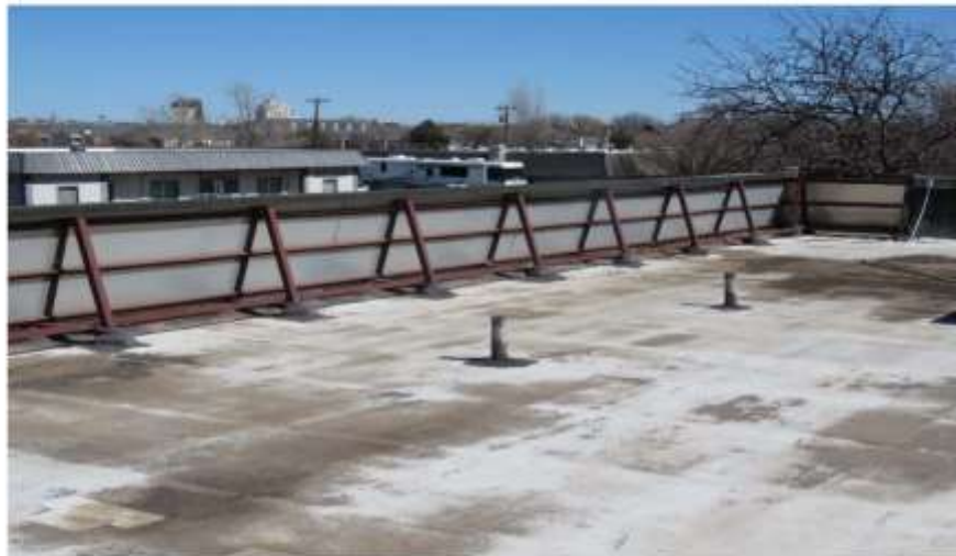
Photograph 13: Interior elevation of the faux parapet-walls on the west, north and east-sides of the building.
