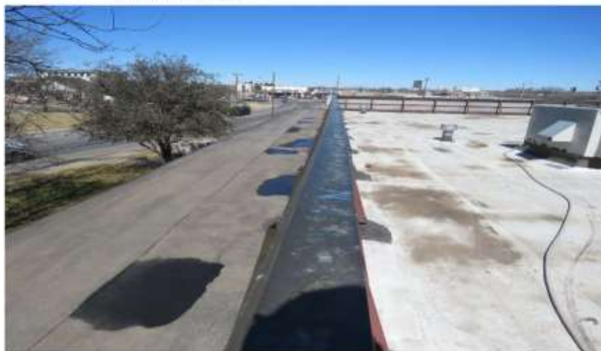
Photograph 32: The field of the modified bitumen membrane is painted with an elastomeric paint from the parapet-walls to the inside of the copper-paneled, faux parapet walls.
