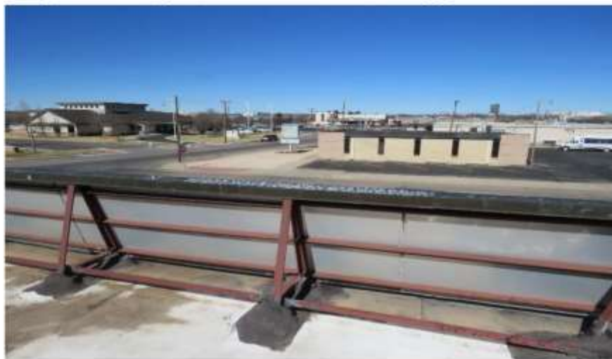
Photograph 38: The copper-paneled, faux parapet-walls frames, which are attached to the surface of the modified bitumen membrane roof, are not displaced.
