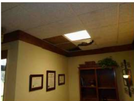
RECEPTION AREA CEILING DAMAGE
