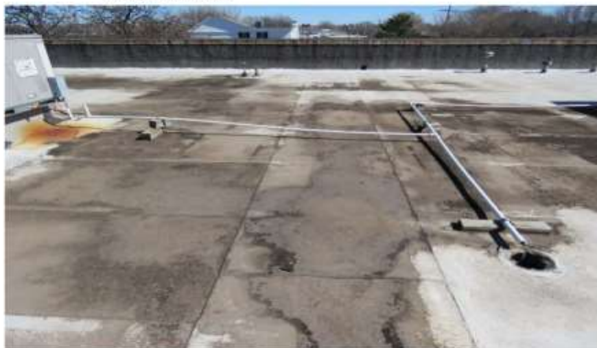
Photograph 40: The paint-covered, modified bitumen membrane has large patches of dark stains with dirt on north of the roof.
