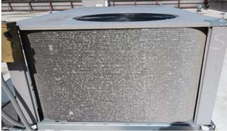
Photograph 19: The HVAC unit's cooling fins are dented.
