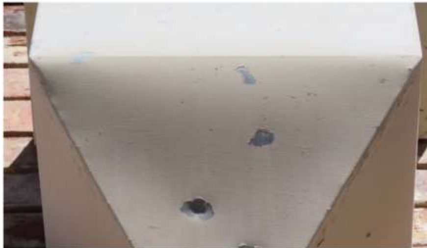
Photograph 5: The scuppers for the roof are dented.
